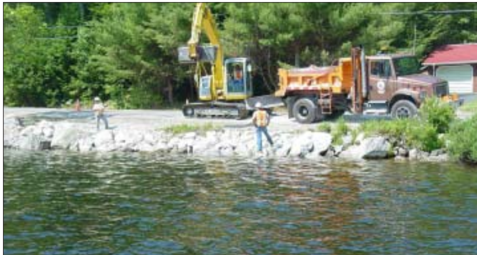
Dan Vining, commanding the excavator, gingerly places fill on the shore of the Landing in Oxford. (Photo: Bob Tracy)
